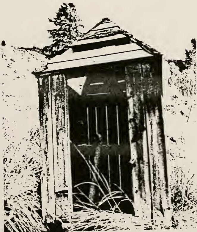
Figure 175. Small wood frame steam pipe shack, located north of Assay office (structure #58) and east of Arsenic plant (structure #59).
